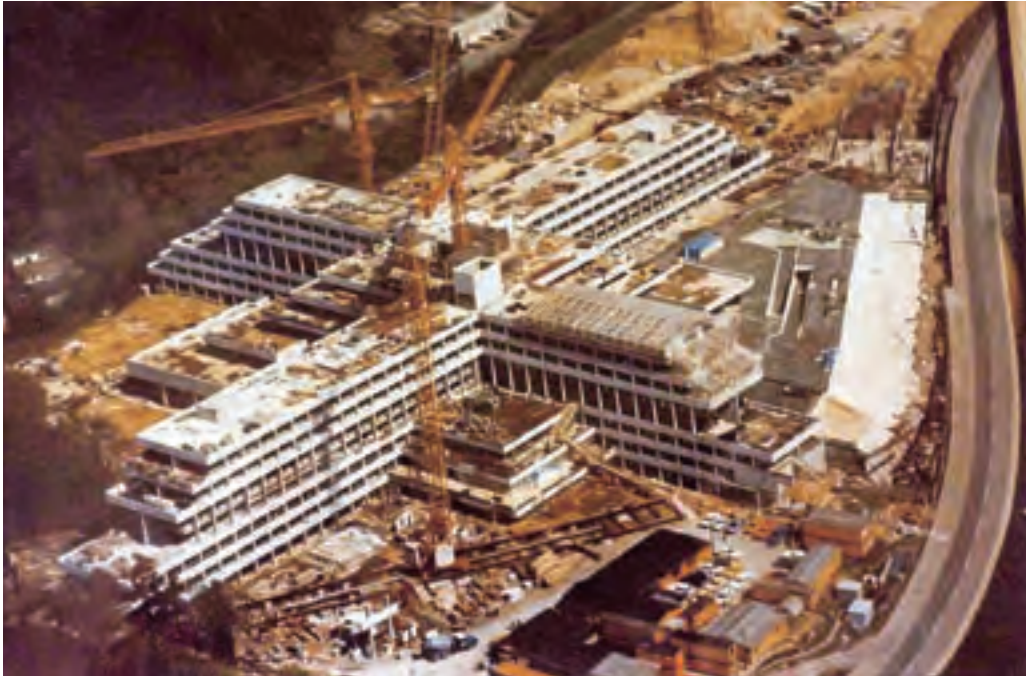
The Kirchberg building site was quite an achievement by the workers. Sometimes they worked day and night to catch up on the huge delays.
