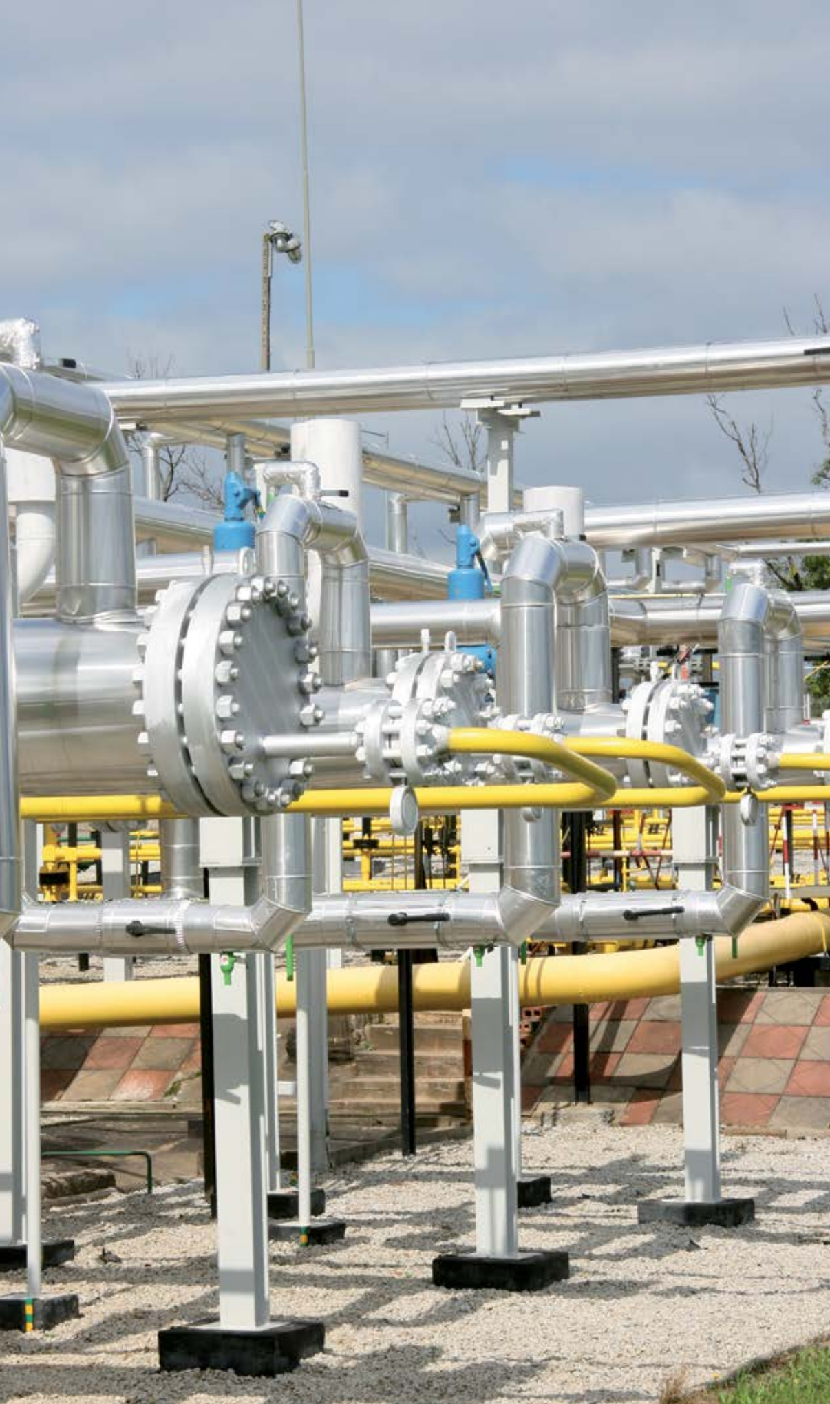
Extension of underground gas storage in Wierchowice, Poland
