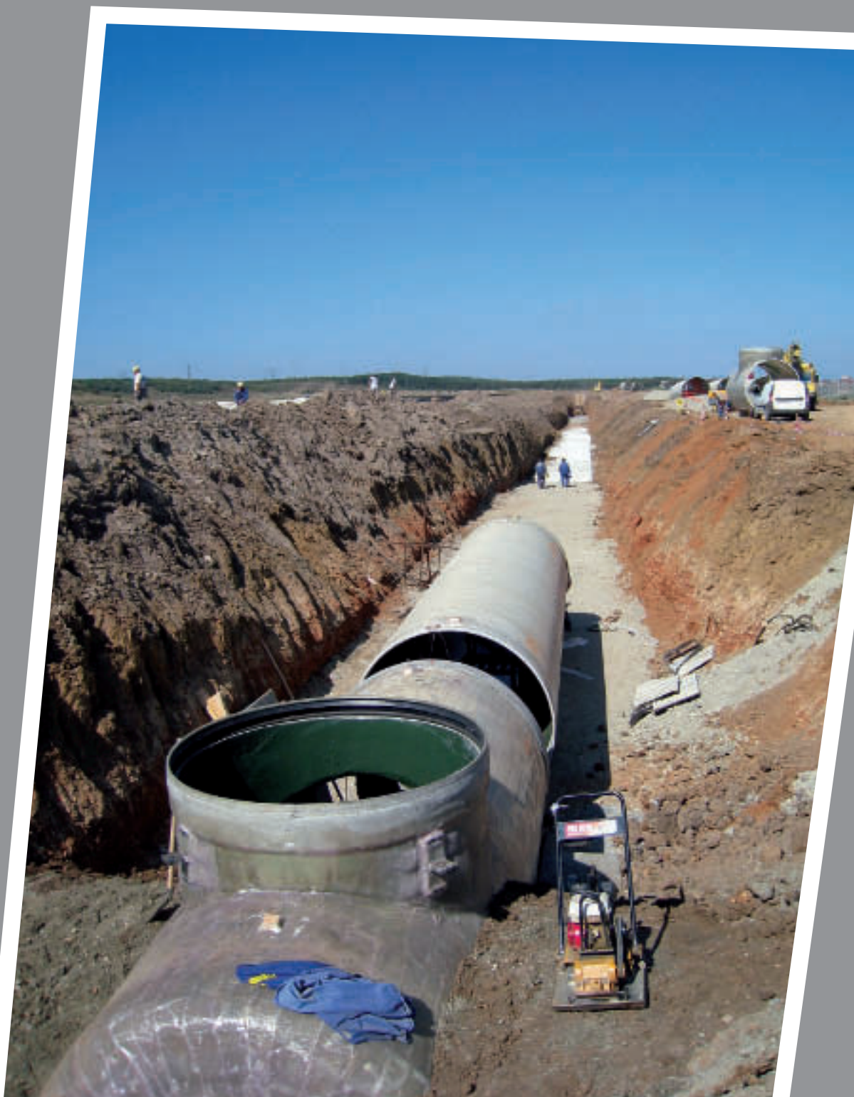
Integrated waste management, Arges, Romania.
